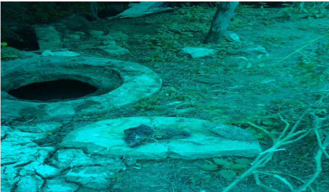
Figure 3: Showing one of the biodigesters with cracked man-hole covers by one of the households that installed biodigesters
