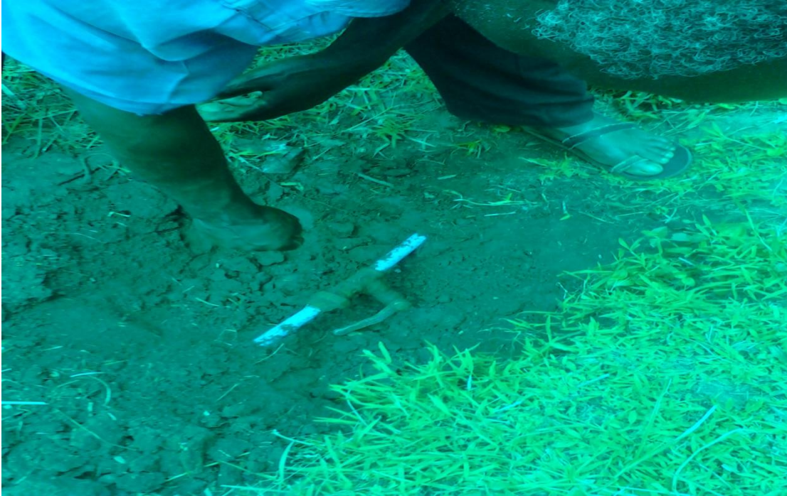
Figure 4: Showing the nature of plumbing works by one of the pioneer households that installed a biodigester in Rukungiri
