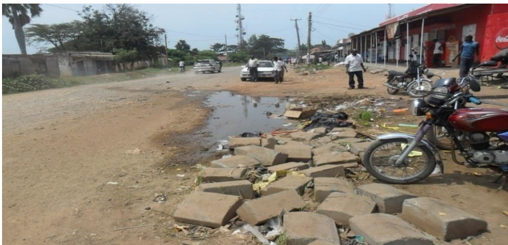
Figure 4: Stalled USMID Road Section in Soroti Town
