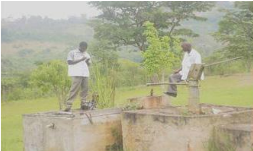
Figure 2: A non-functional hand pump in Tirinyi in Kibuku District
